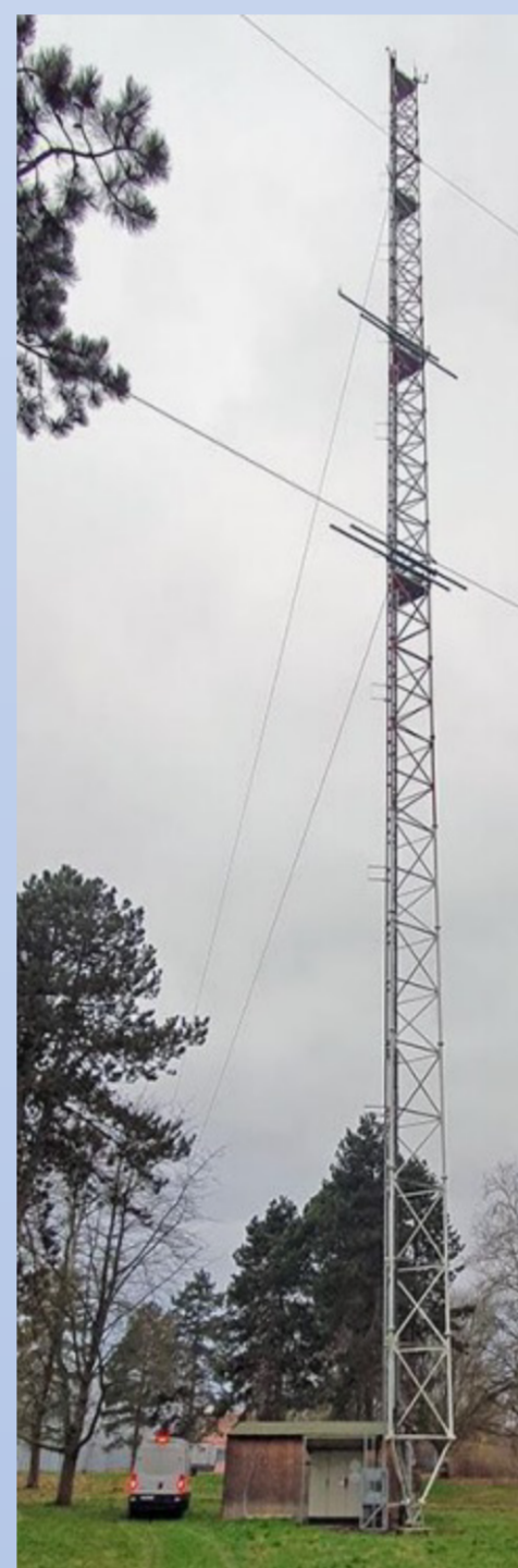
Tower and shelter at Saclay ICOS station.
